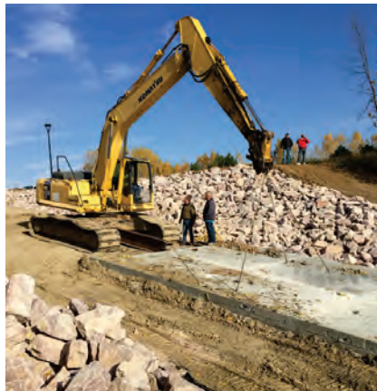
Rutjens Construction slides a section of the new boat ramp into the water.
