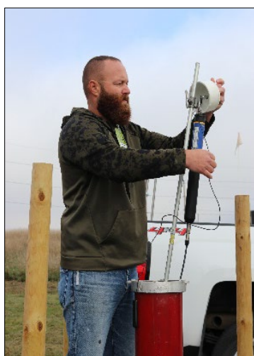
Monitoring Well – Platte County NRD Realtime Telemetry
